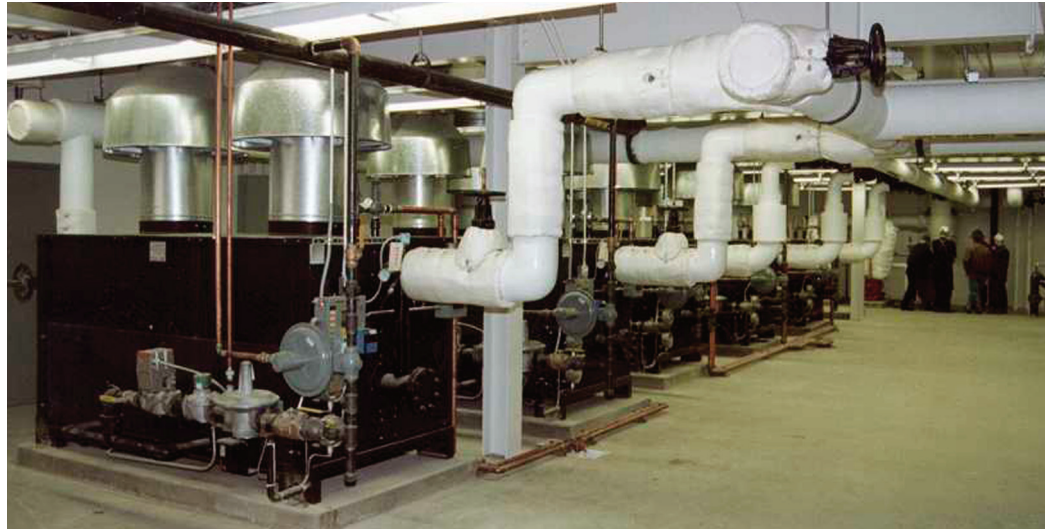
The Parker bent steel tube, all welded construction is the ideal boiler for high temperature applications. Pictured is the Boiler Room at HMT Technology Corp. in Eugene, Oregon. Here, two T-4600's provide the heat source for a metal plating line (350°F), and three T-6800's serve the building heating needs of the facility.
